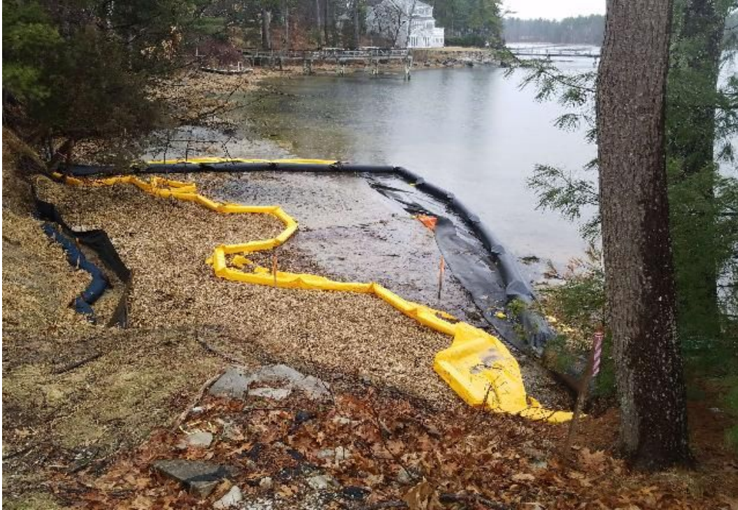
Fig 1: Turbidity curtain in intertidal zone at Gundalow landing/east side of the Bay. Viewing south. (03-19-20).
