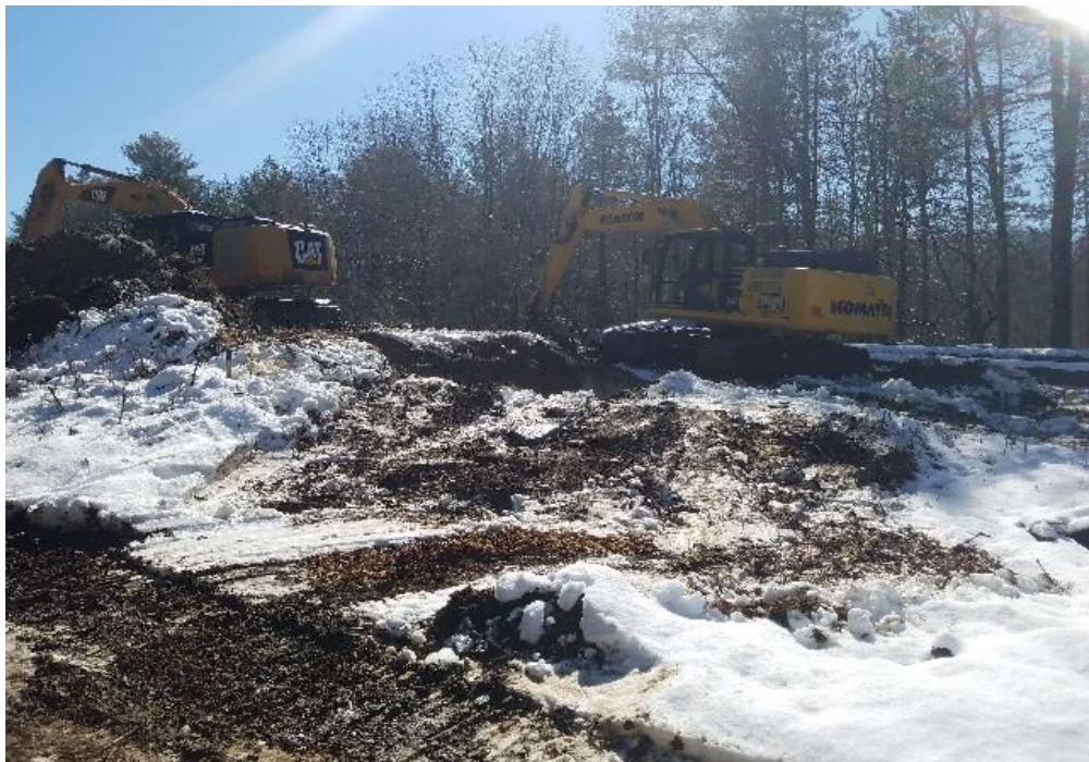
Fig 14: Hammering ledge at Str. 75. Viewing southeast. (03-24-20).
